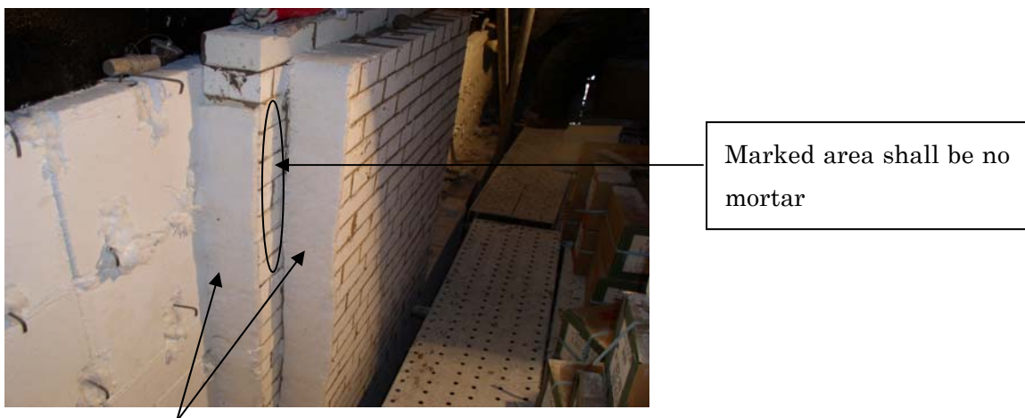
Expansion Joint with C/F Blanket
